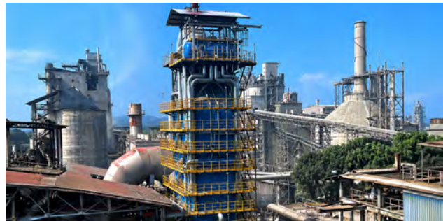
YTL-APMC Waste Heat Power Generation
